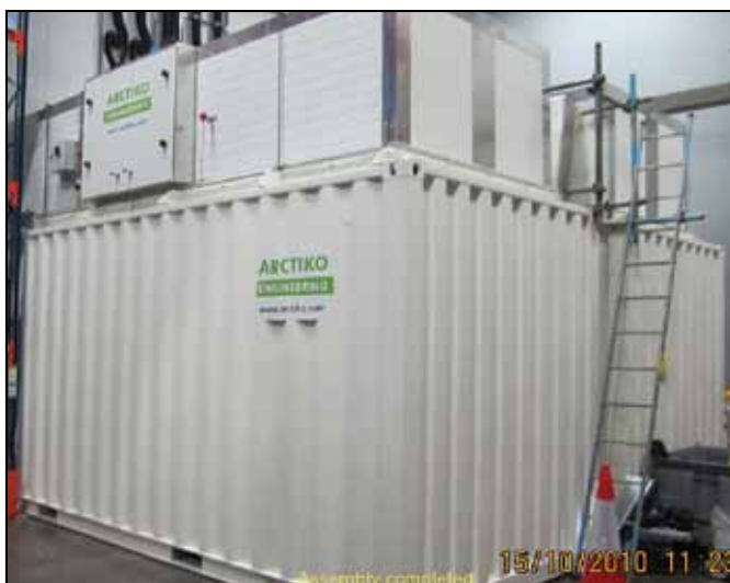
Picture from the installation in late 2010.
